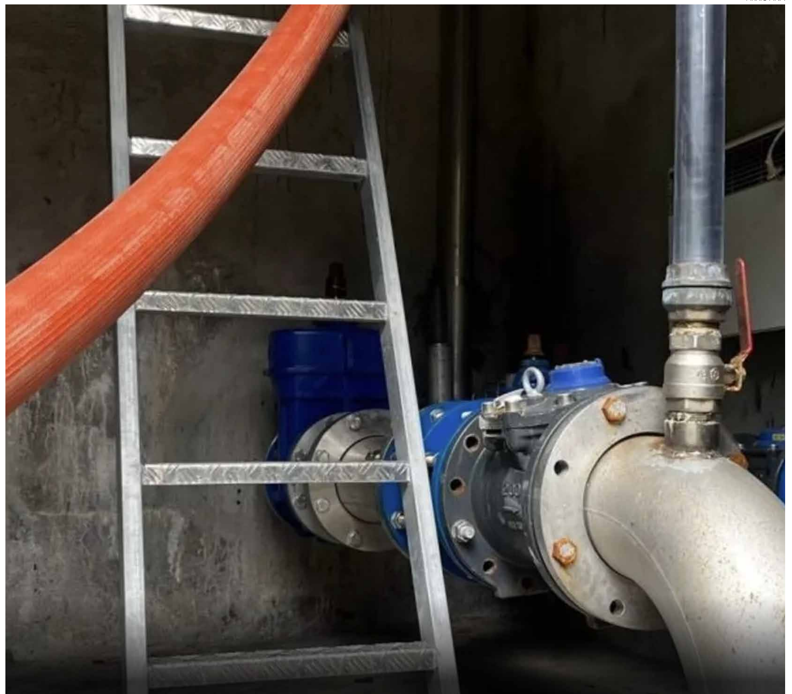
A water tank.
